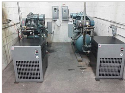
MHT130 HIGH TEMPERATURE AIR DRYERS INSTALLED IN LIVONIA, MI
